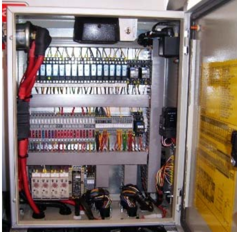
Mallaghan Sample Electric Fuse Box
