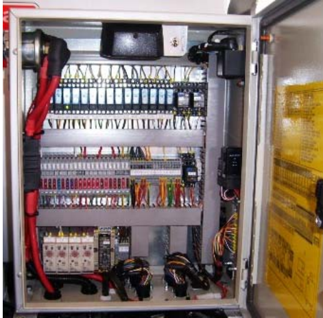
Mallaghan Sample Electric Fuse Box
